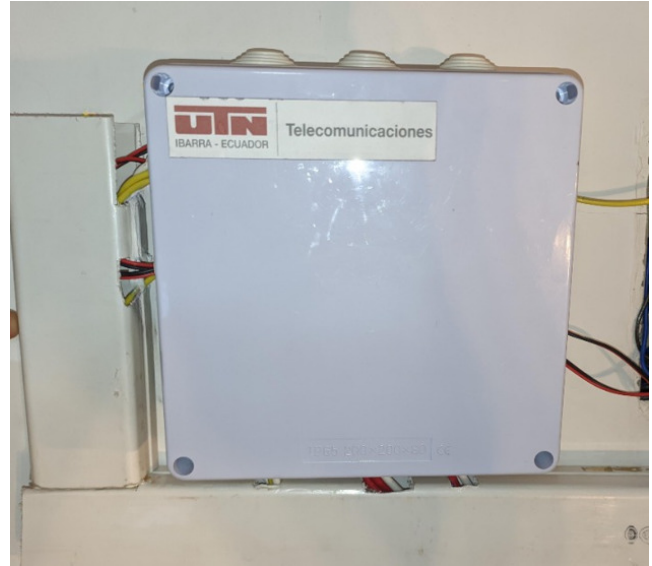
Figure 13. Node 2 Deployment (Distribution Panel)
