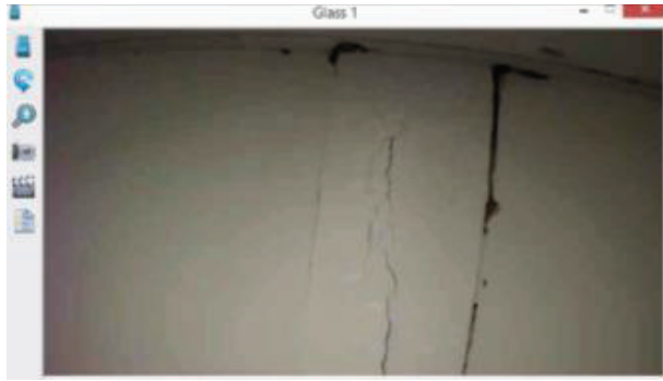
Fig. 23. Operator's vision while performing a structural inspection task using the AR.Drone (image captured from Glass screen using Droid@Screen application).
